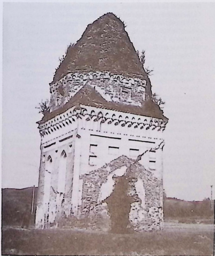
Plate 29. A gunbad south of Sari, damaged by the 1935 and earlier shocks.
